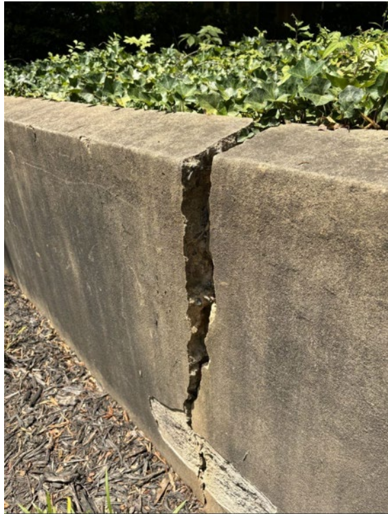
Left side wall with damage
