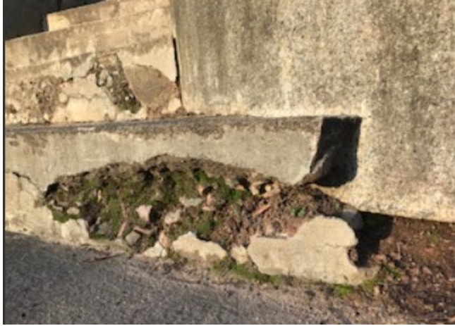
Damage to stair risers
